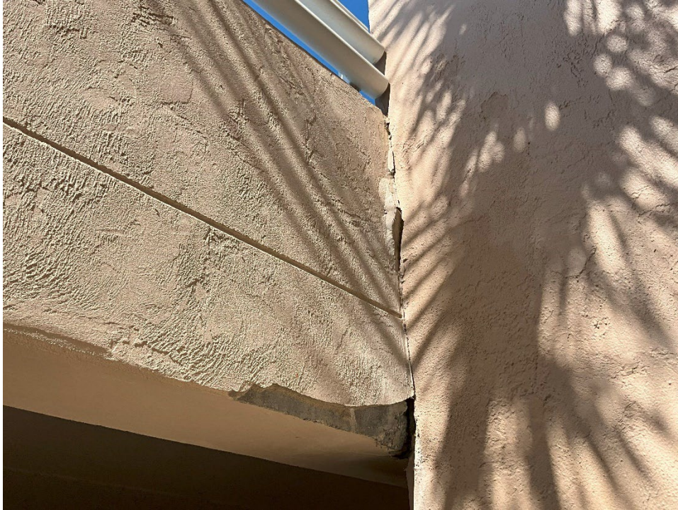
52. The portion of beam where the Parking Deck intersects with the Elevator Tower wall is spalled and EIFS system is cracking off at the joint due to water intrusion.
