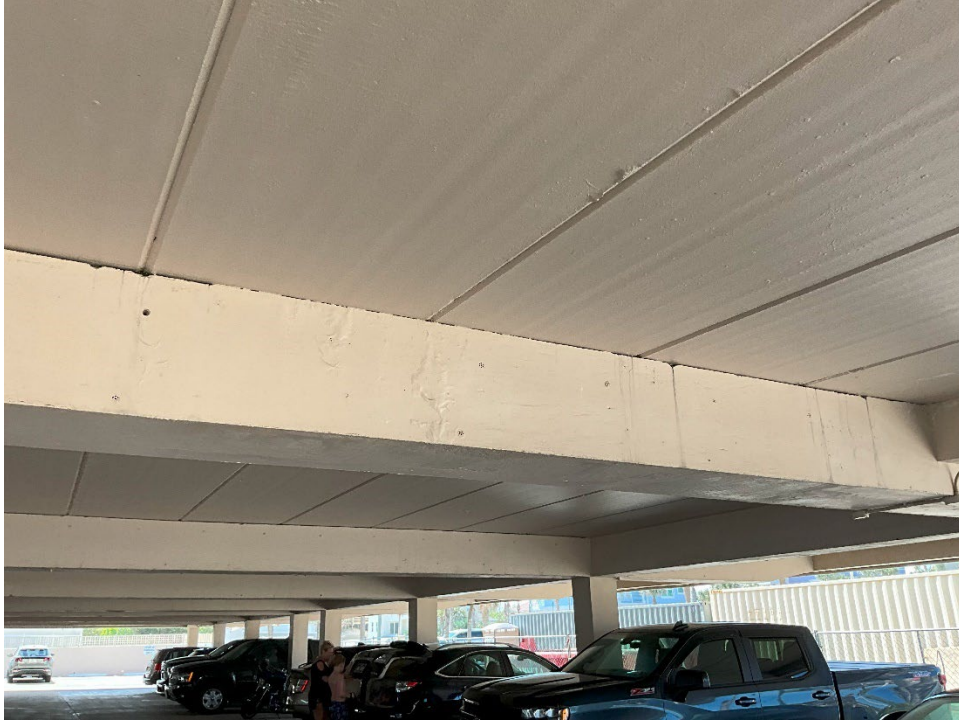
49. Additional water intrusion along the beam under the Parking Deck.
