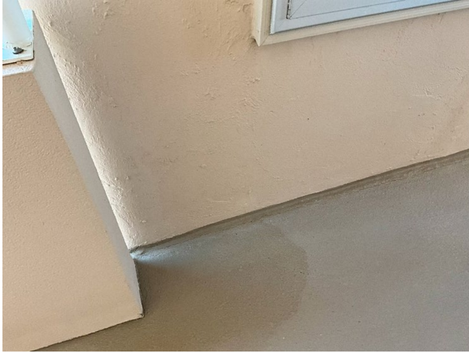
19. View of the cracks along the joints between the floor and the wall outside of Unit 501.
