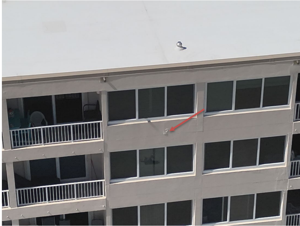
13. View of the additional area of the northeast wall at floor 7 where water infiltration is occurring.
