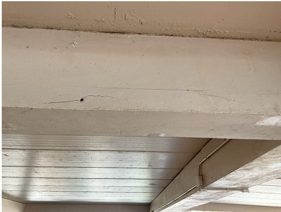
46. Additional tensile cracks along beams in Parking Deck. The paint and stucco will need to be removed to expose the beam for Phase II.
