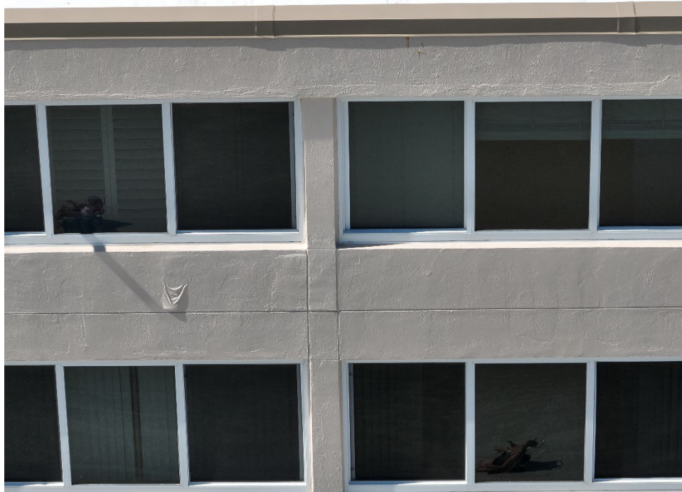
14. View of the additional area of the northeast wall at floor 7 where water infiltration is occurring.
