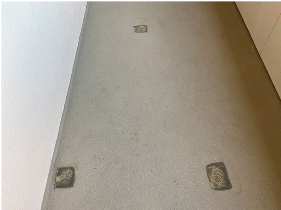
40. Patches in the Breezeway floor outside of Unit 104.
