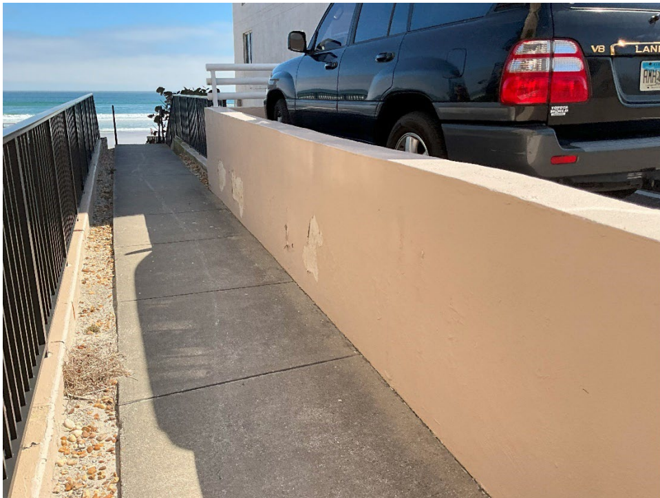
56. Paint delamination noted along the wall next to the beach access sidewalk.
