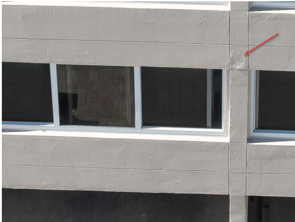
16. View of the additional area of the northeast wall at floor 1 where possible water infiltration is occurring.
