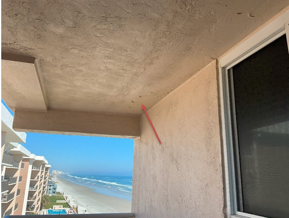
35. Paint delaminated paint is shown on the ceiling of Breezeway outside of Unit 601, 602.
