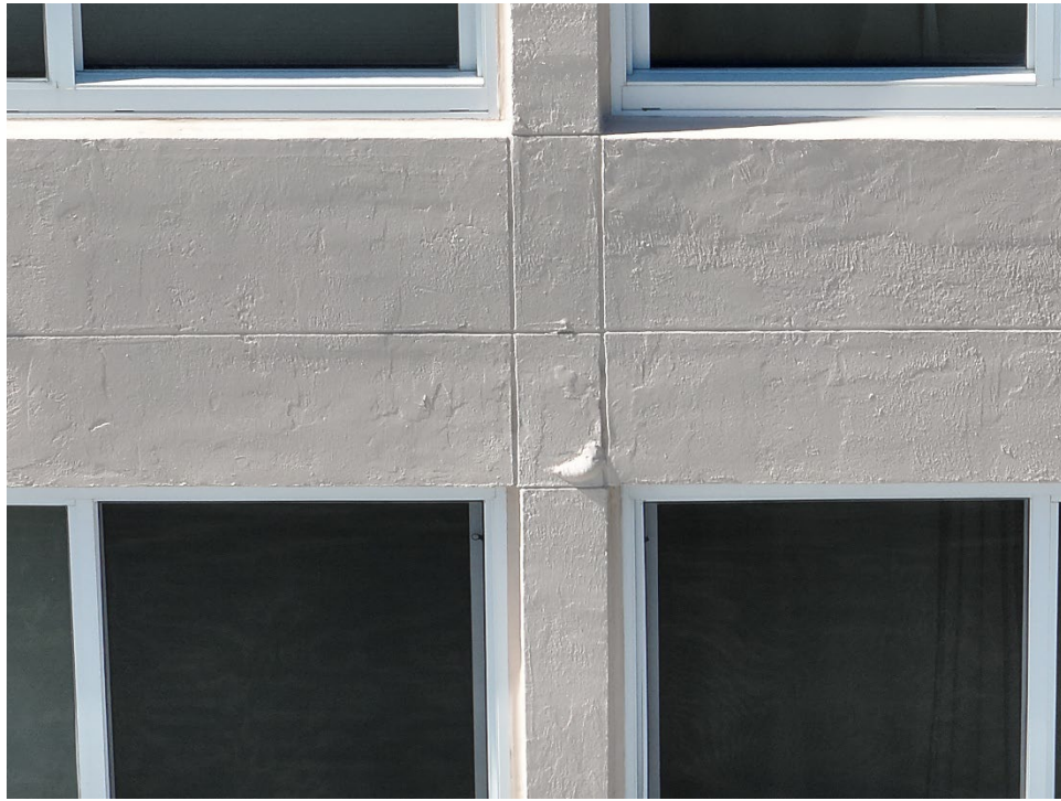
15. View of the additional area of the northeast wall at floor 6 where water infiltration is occurring.
