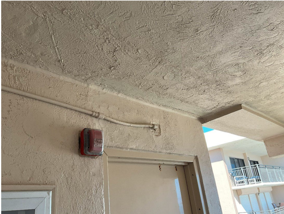
58. Typical example of the fire safety equipment installed.
