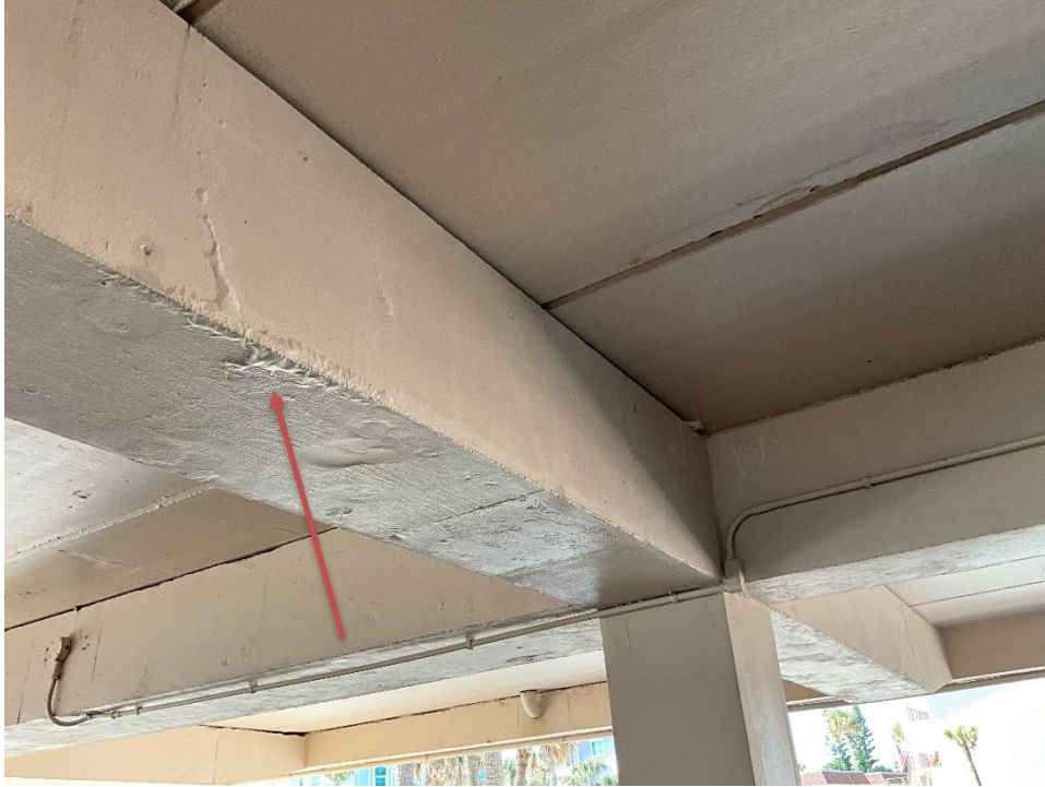
47. View of water intrusion along the beam under the parking deck.
