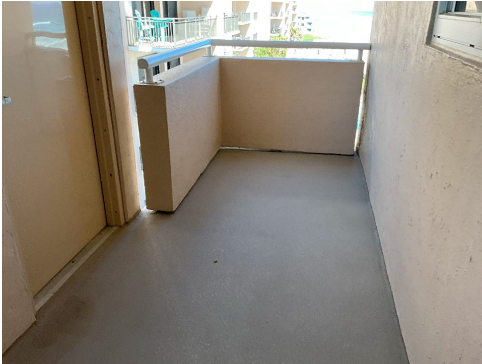
34. View of the parapet wall constructed out of plane with a sloped Breezeway outside of Unit 401.
