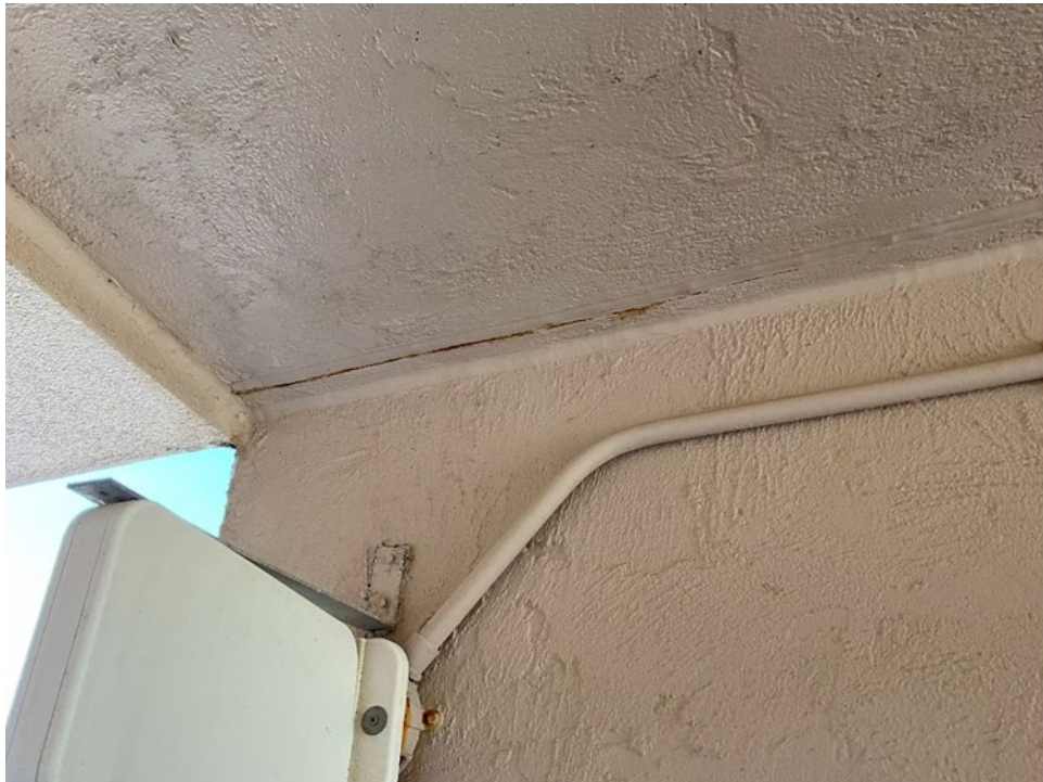
20. View of the cracks along the joint between the wall and the ceiling outside of Unit 501.
