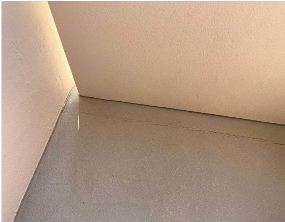
25. View of a crack along the control joint in front of the Breezeway safety wall near Unit 111.
