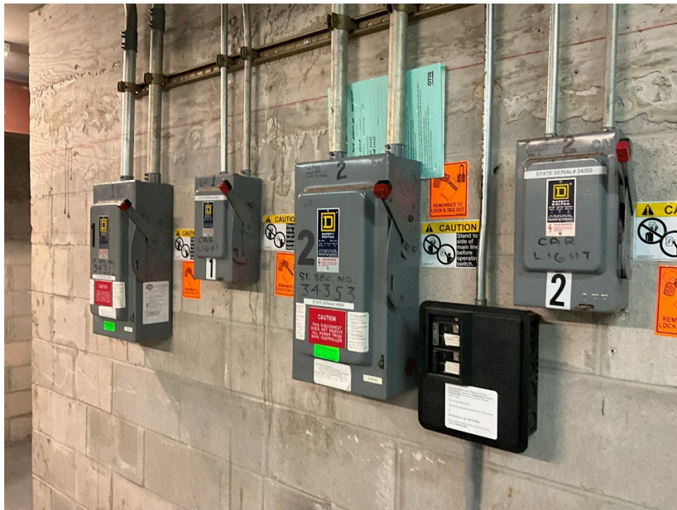
62. An Example of the electrical equipment.
