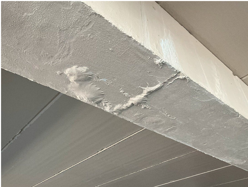
48. Additional water intrusion and efflorescence along the beam under the Parking Deck.
