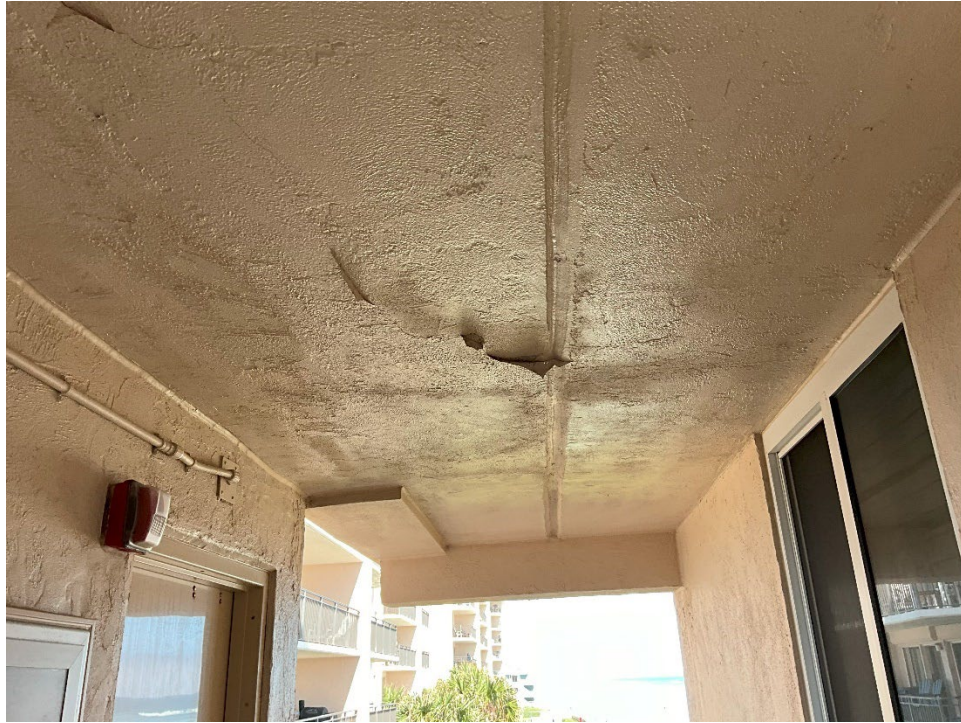
39. Additional paint delamination on the ceiling outside of Unit 201.
