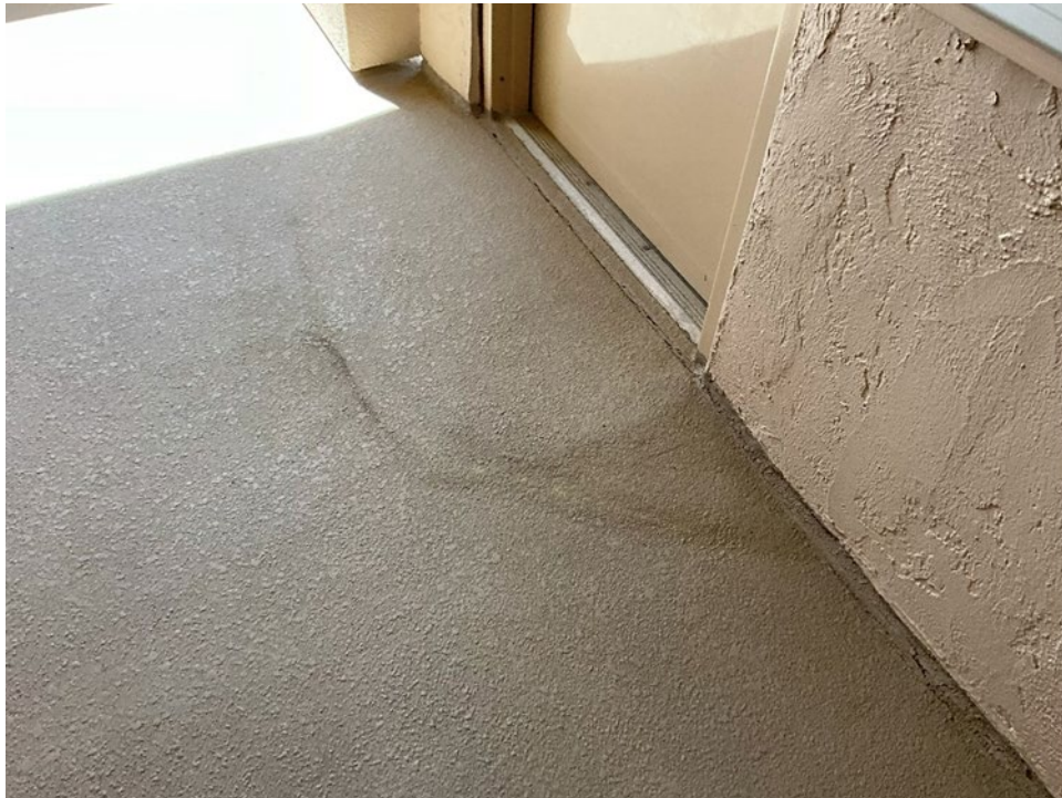
24. View of cracks and staining from water ponding on the slab in the Breezeway outside of Unit 110.
