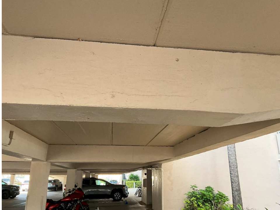
45. Tensile crack in beam under Parking Deck. The paint and stucco will need to be removed to expose the beam for Phase II.
