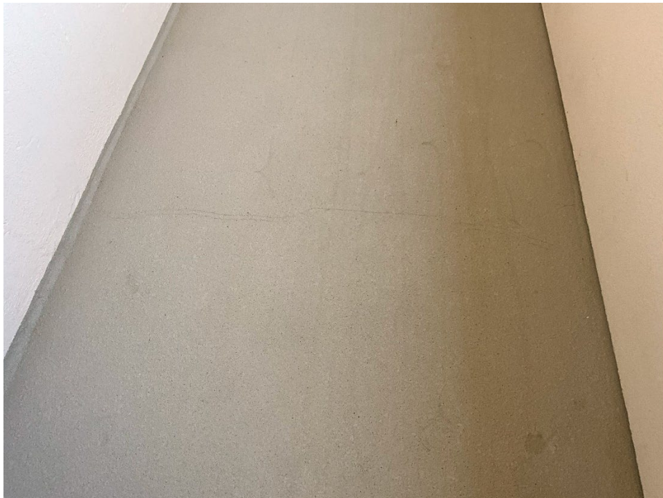
26. View of the cracks along the missing control joints in the breezeway along the hallways of each floor.
