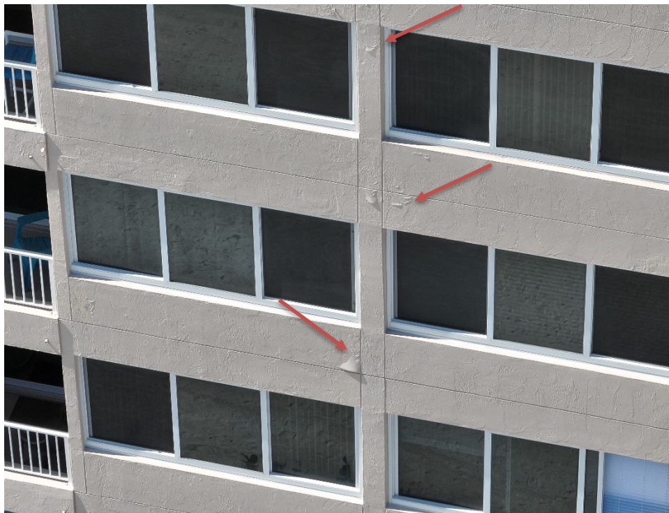
12. View of the areas of the northeast wall at floor 4 and 5 where water infiltration is occurring.
