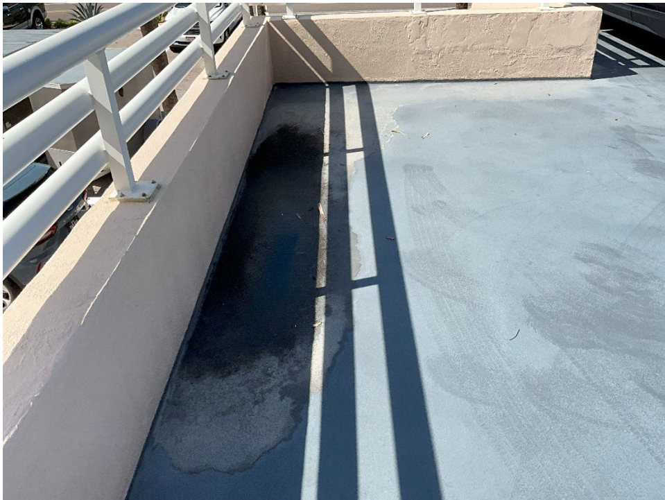
54. View of water ponding and paint delamination on the top level of the Parking Deck.
