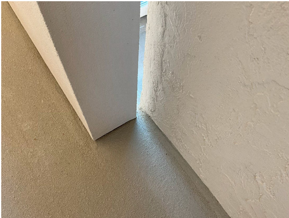
18. View of the cracks occurring along the control joint in the corner where the Breezeway wall meets the Elevator Tower on the 7 th floor, outside of Unit 501.
