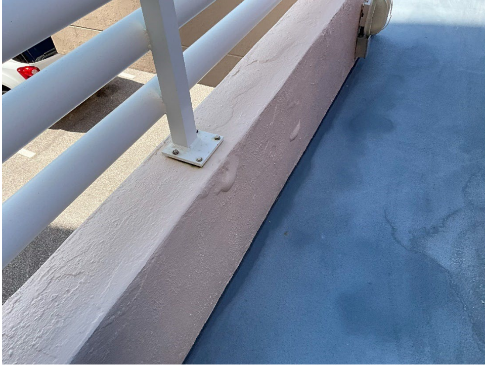
53. View of water intrusions showing in the wall of the Parking Deck.
