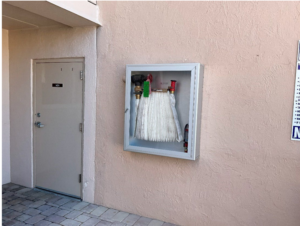
59. Additional typical example of the fire hose equipment installed.
