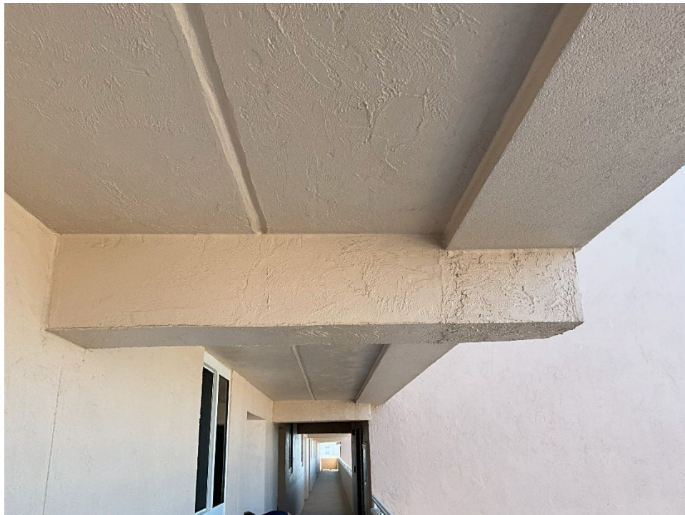
30. View of the previously patched beam outside of Unit 504.
