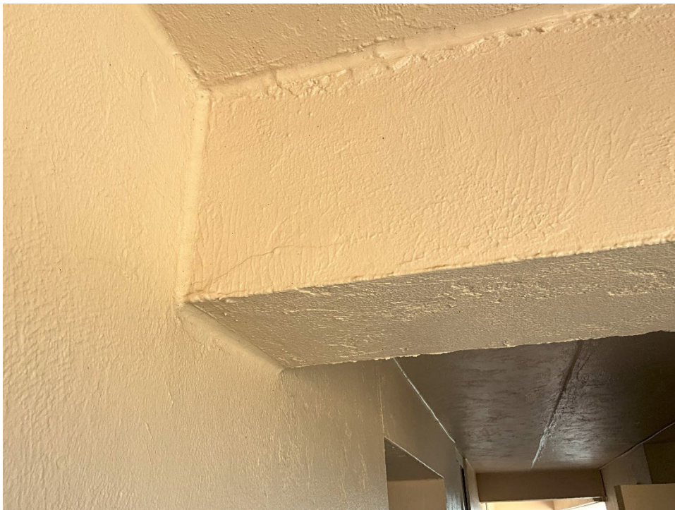
28. A tensile crack is shown running along the bottom of the beam outside of Unit 704.
