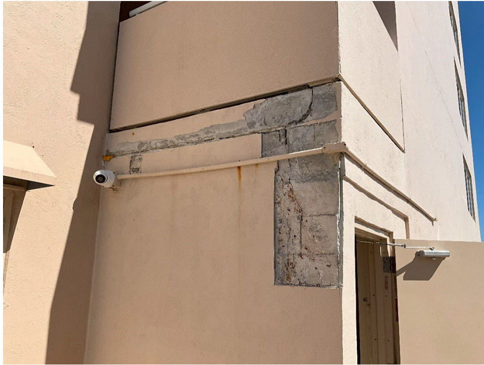
41. Exterior shear crack in CMU wall with removed EIFS system. Perform Geotechnical testing to investigate evidence of settlement for Phase II.
