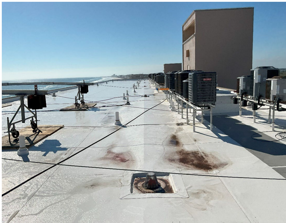
4. Additional photos of the entire roof system with a flat roof membrane.
