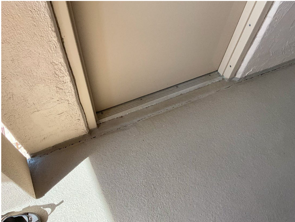
22. View of cracking along the joint between the floor and the wall outside of Unit 211.
