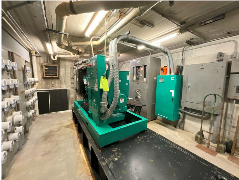
61. Typical example of the generator equipment.
