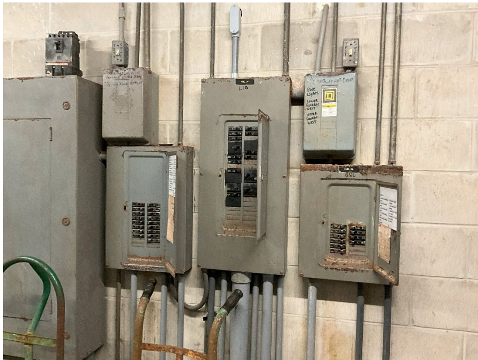
60. Typical example of the electrical equipment with corrosion.
