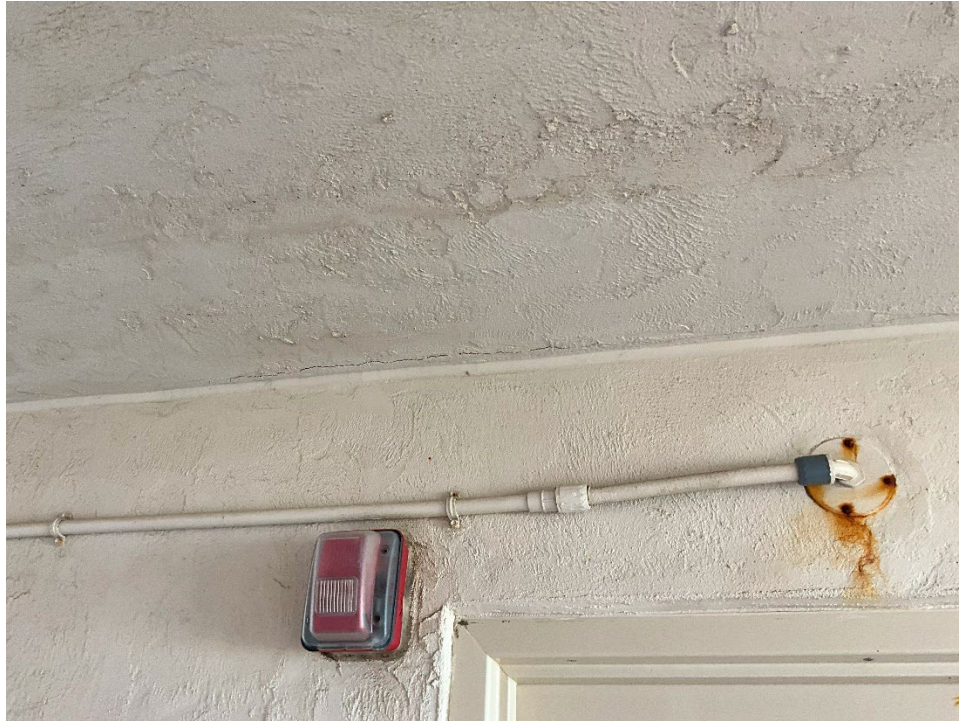
23. View of cracking along the joint between the ceiling and the wall outside of Unit 101.
