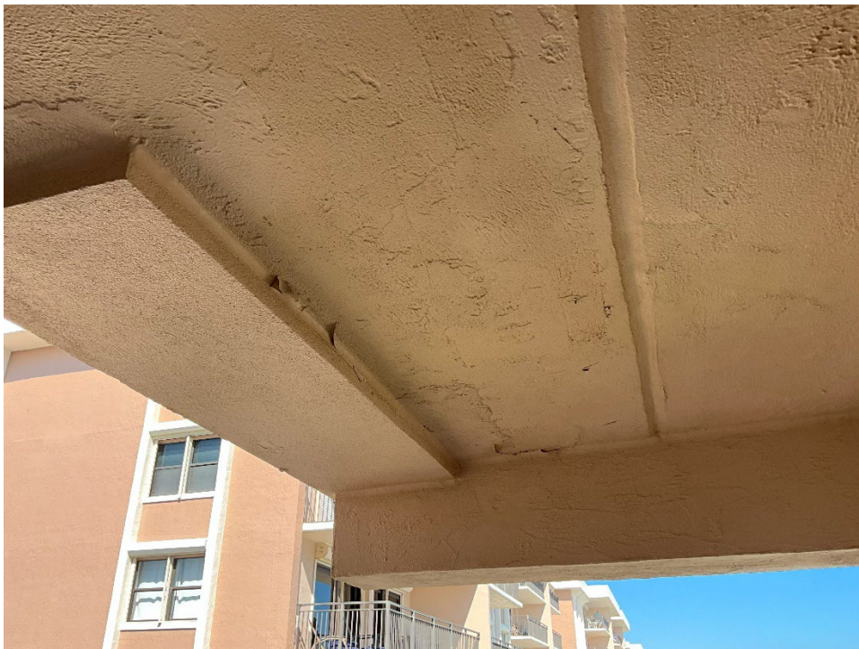
36. View of paint delamination on ceiling outside of Unit 401.
