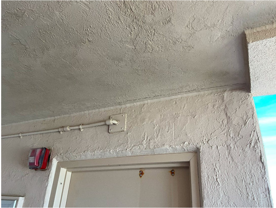
21. View of cracking along the joint between the ceiling and the wall outside of Unit 301.
