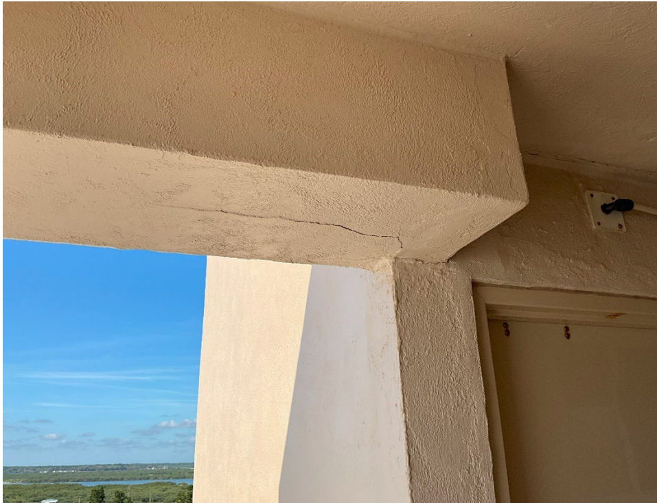
27. View of the Visible cracks along bottom of beam outside of Unit 710. The paint and stucco will need to be removed to expose the beam for Phase II.
