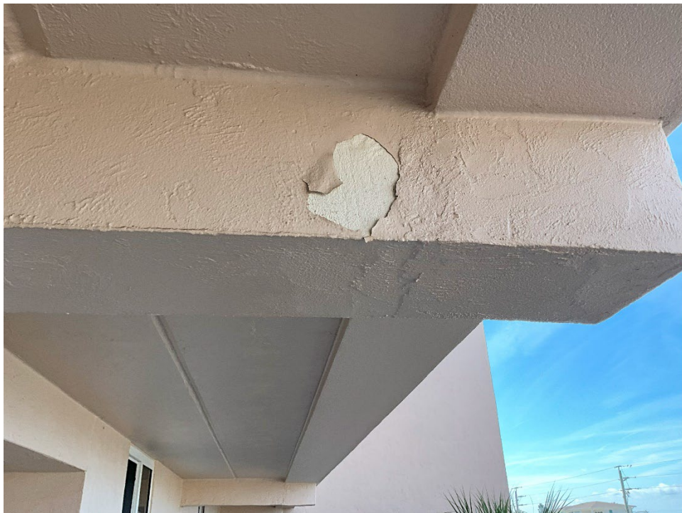
38. View of paint delamination on beam outside of Unit 204.
