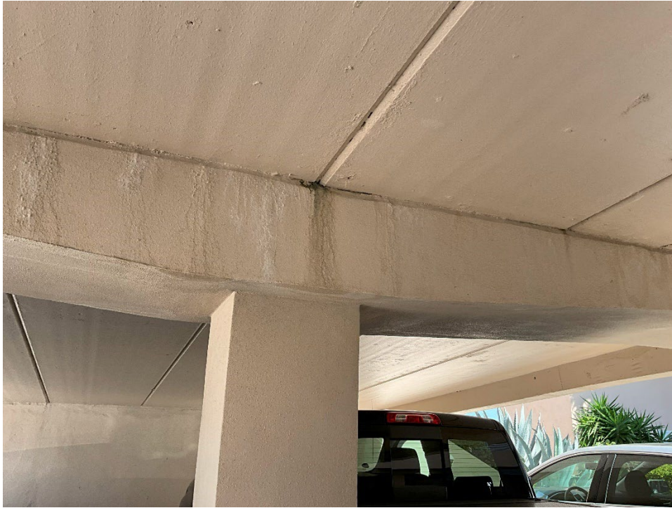
51. Additional efflorescence shown on beams under Parking Deck.
