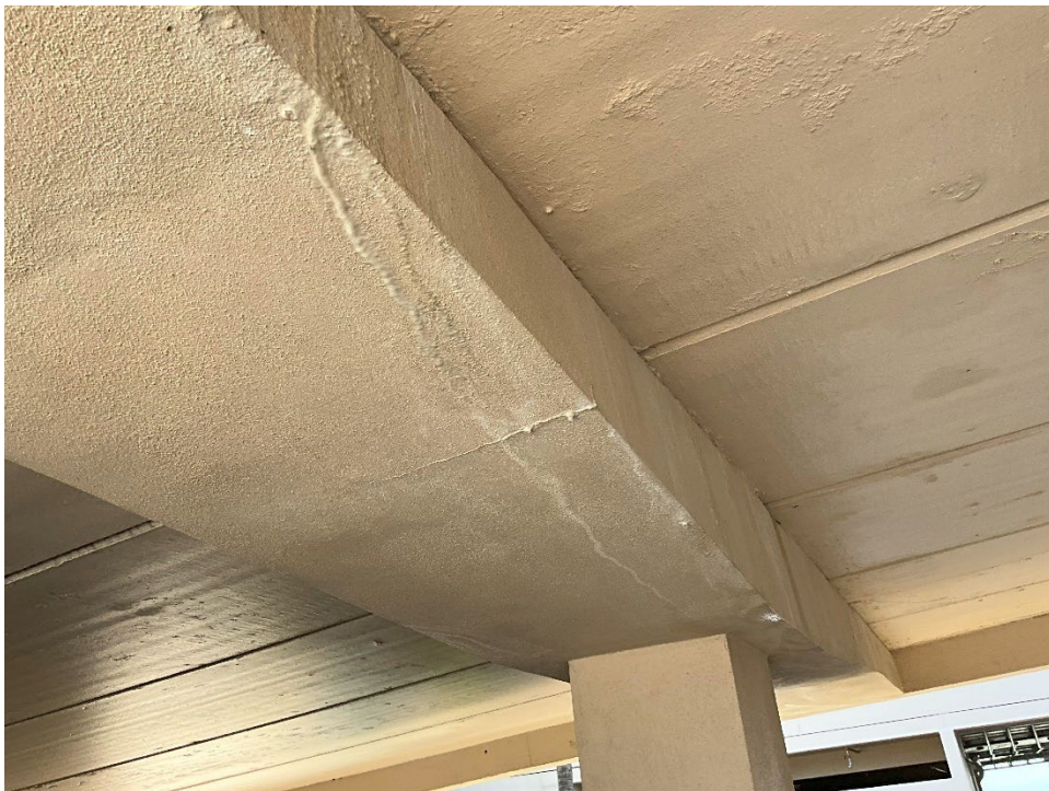
50. Efflorescence is evident under the beams under the Parking Deck.
