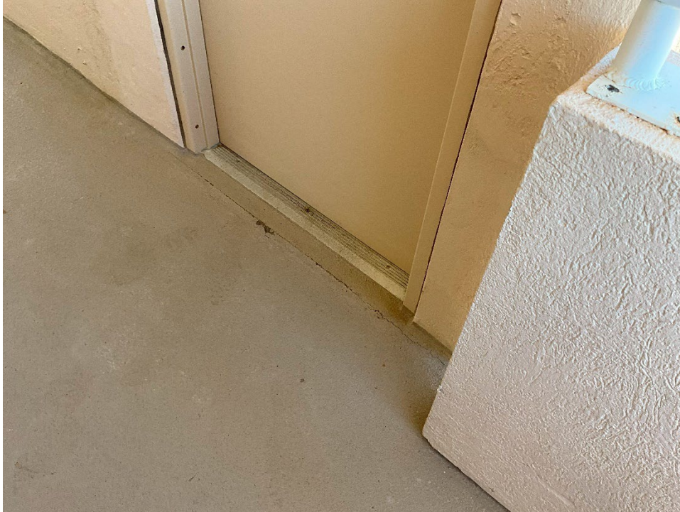
17. View of the cracks occurring along control joint in front of the door to the Elevator equipment room on the 7 th floor.
