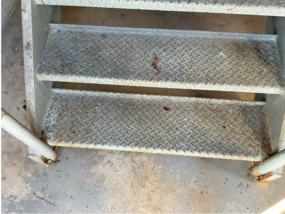
57. View of the bottom of the stairs, located in the Elevator Tower, are showing signs of corrosion.
