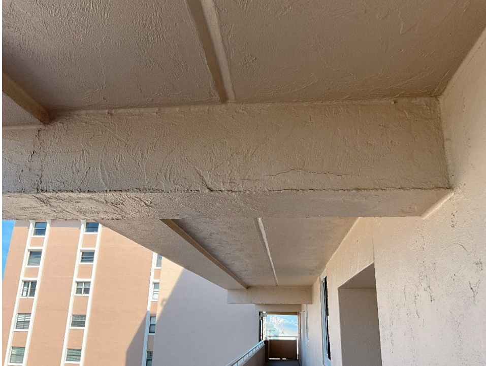
33. Tensile crack along bottom of beam outside of Unit 404. The paint and stucco will need to be removed to expose the beam for Phase II.
