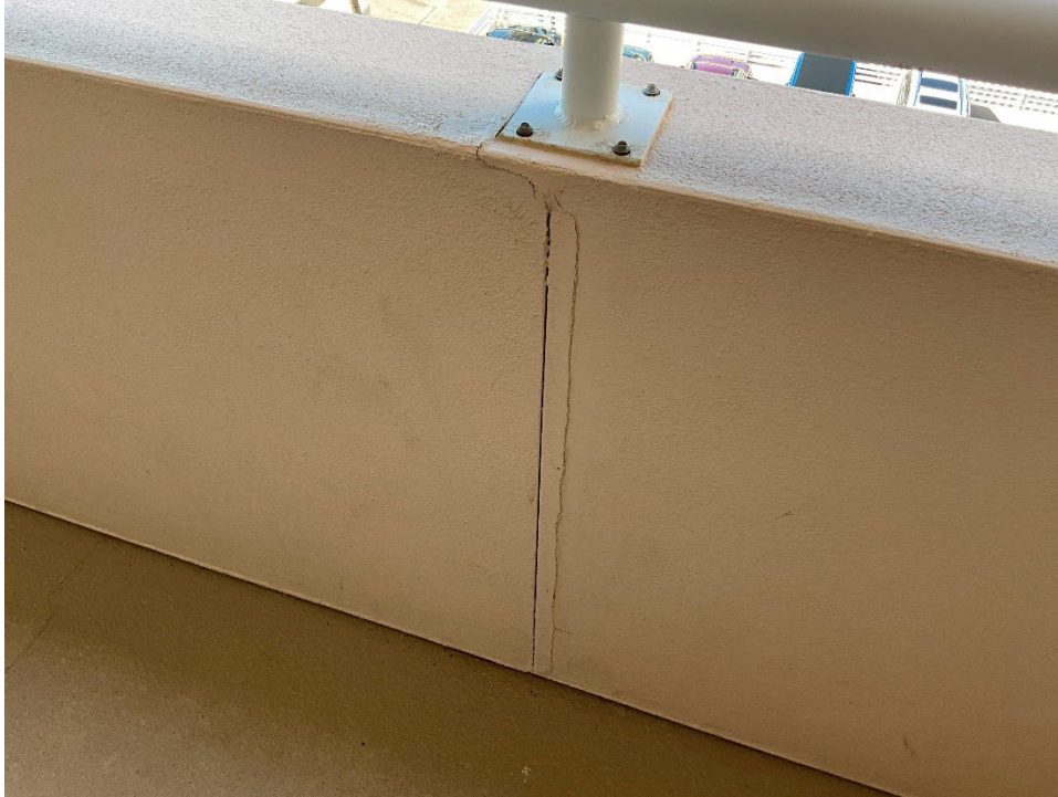
31. View of the crack in the parapet wall next to the control joint outside of Unit 507.
