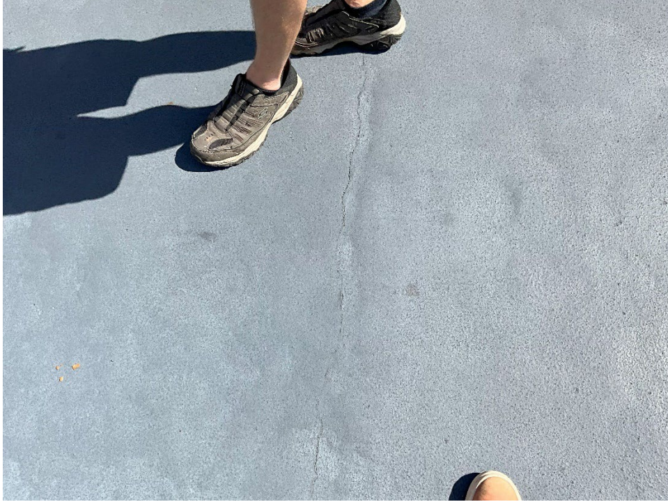
55. Cracks along the expansion joints in the Parking Deck.
