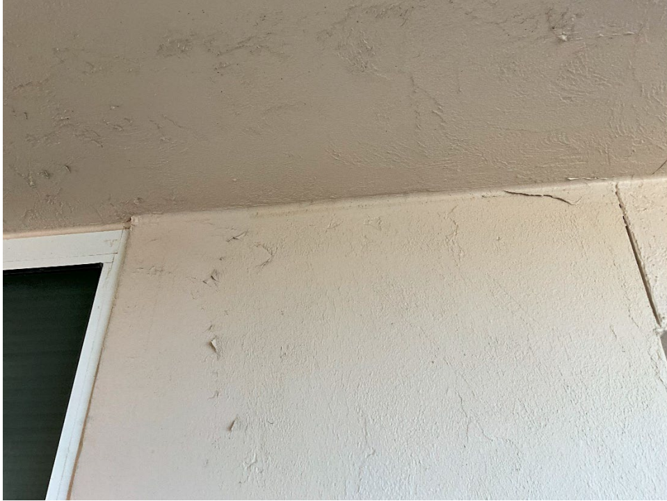
37. Additional paint delamination on the wall outside of Unit 301.
